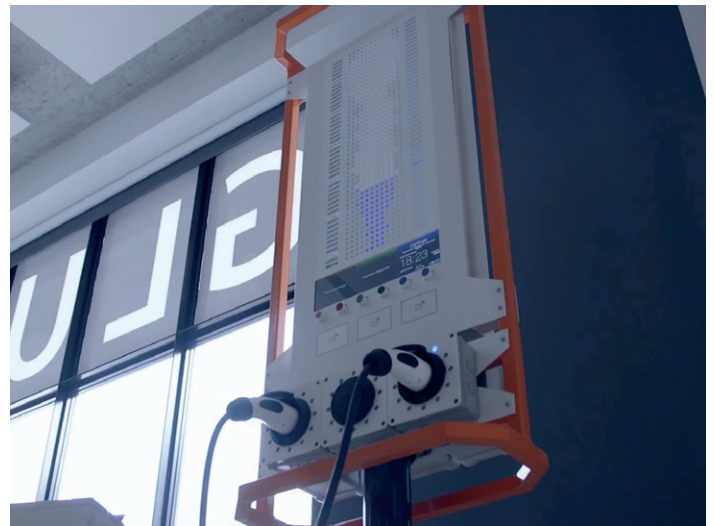
The transparent charging station from Alliander (Photo: Alliander)
